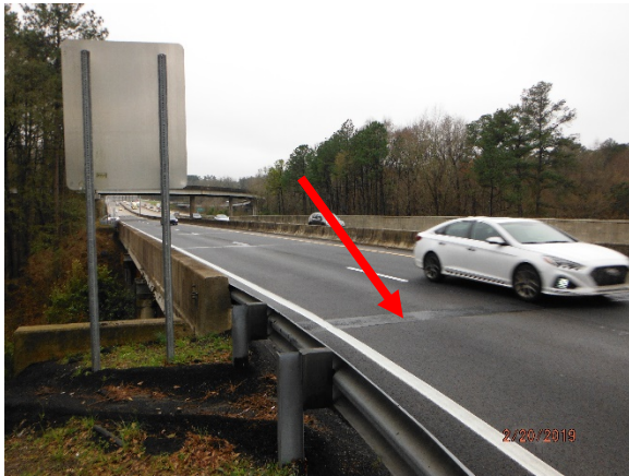
Photo 3. Black Mastic on Asphalt Overlay at Expansion Joints
