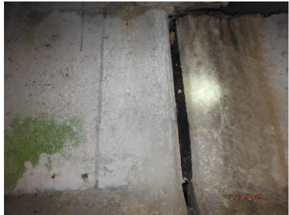
Photo 4. Black Expansion Joint Material
